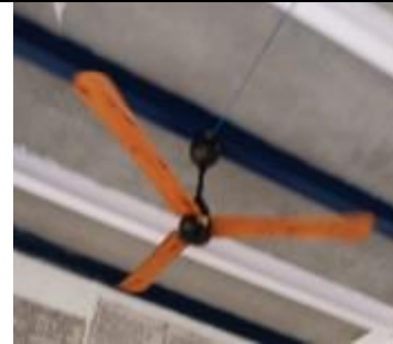
3 New power saver fans fitted. 12 more required
