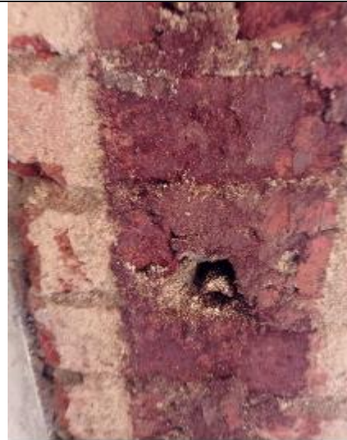
Live termite found in wall
